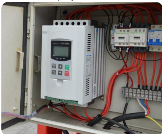
Soft Start to protect electric motor
